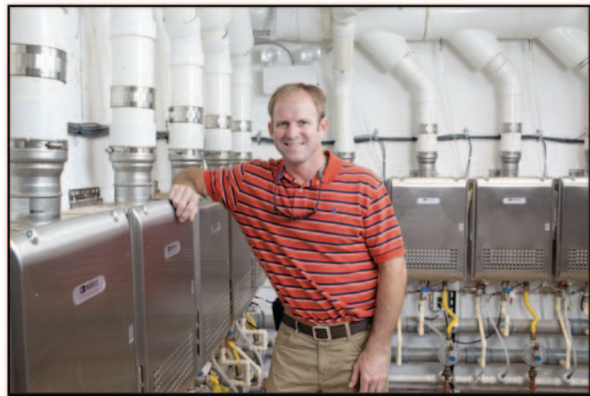
Jason Veal of the Tallman Company, shown with the tankless water heater installation at the Residence Inn in Florence, Ala. According to Veal, he and contractor Anthony Crouch “told the hotel owner that we could make it work — barely.”
