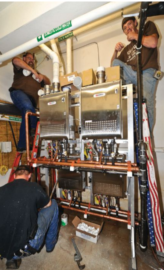
Members of a local plumbing crew put the finishing touches on a rack assembly in a restaurant mechanical room. Beyond the tankless rack installation, FRG makes sure every hot water usage point in a restaurant operates properly.
