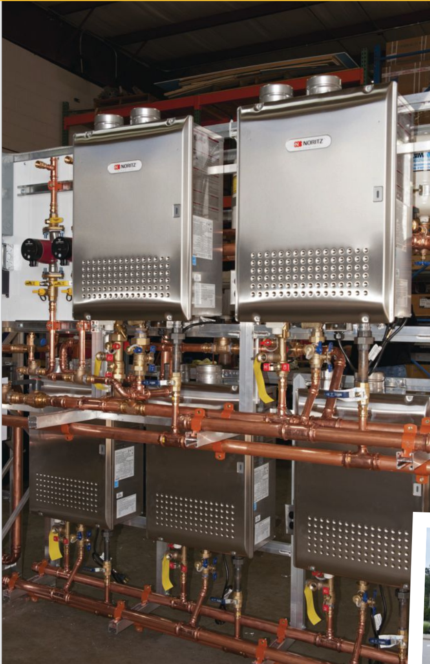
Facilities Resource Group's tankless water heater rack assemblies are designed and fabricated at the company's Grandville, Mich., headquarters and then driven to restaurants for installation.
