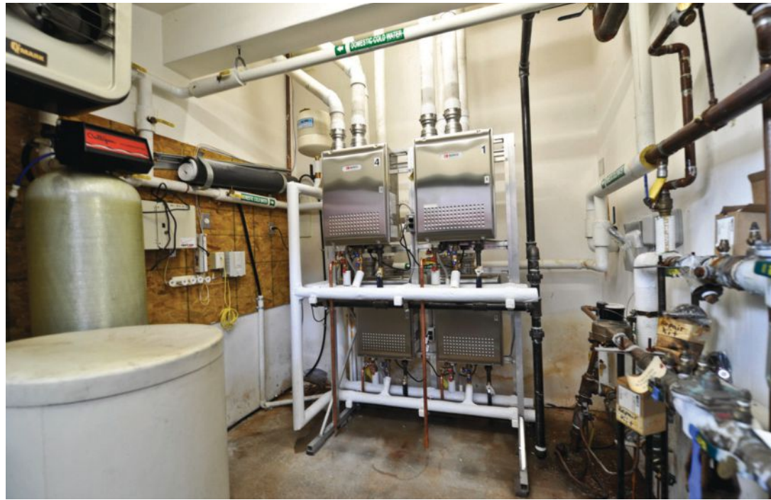
An informal survey of the first rack installation at a PDI Chili's property in 2010 reveals the restaurant saved roughly $1,800 per year in energy costs.
